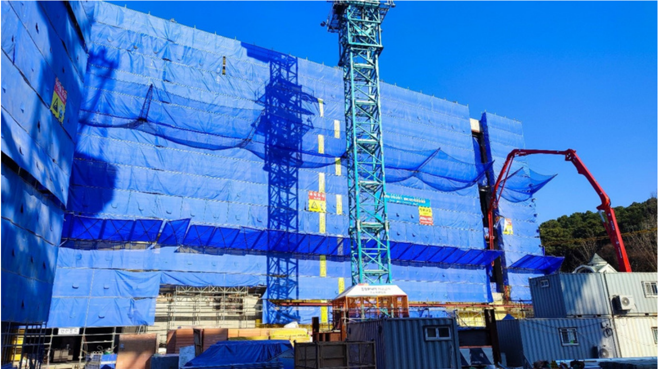
External view of KINX's Gwacheon Data Centre under construction, November 2023 (Source: ICM)
